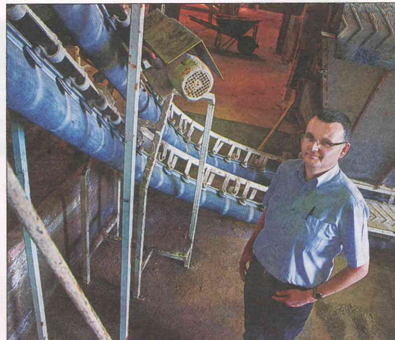
NEW PROCESS: David Bonfield says the ICS conveyor system has made a big difference to production at the Baileys factory.
