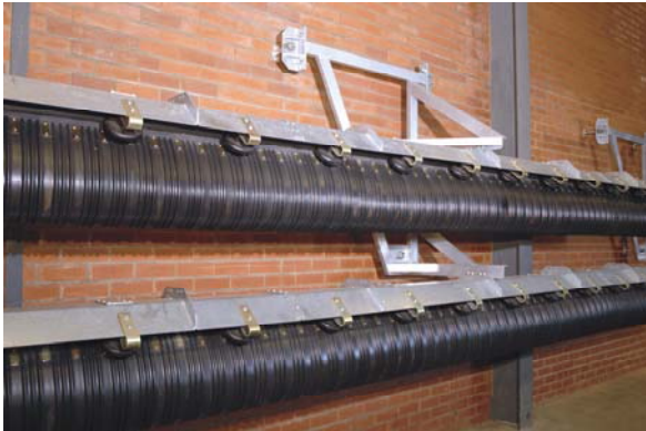
Figure 3: Example of wall mounted frame
