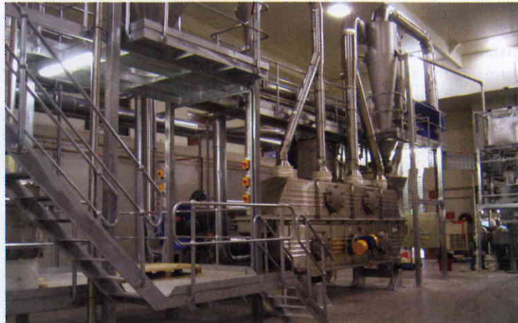
New Food Coatings' factory in Wetherill Park, NSW, recently installed this fluidised bed dryer, supplied by iBulk.
