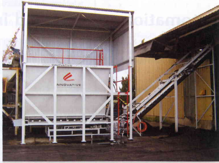
This hopper and conveyer was recently installed as part of a system to convey mulch, potting mix and soil conditioner to a bagging machine inside the plant.
