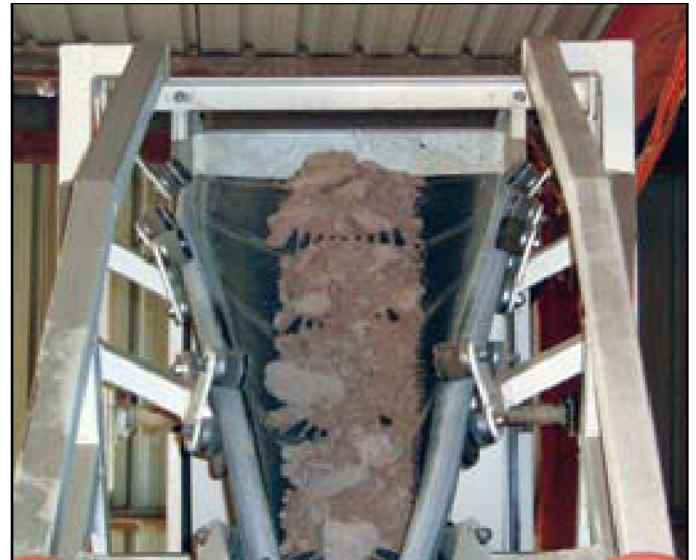
ICS conveying up a 40 degree vertical angle.
