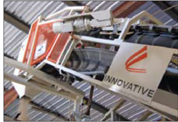
Existing Innovative Conveying System (ICS) at Baileys Fertilisers.
