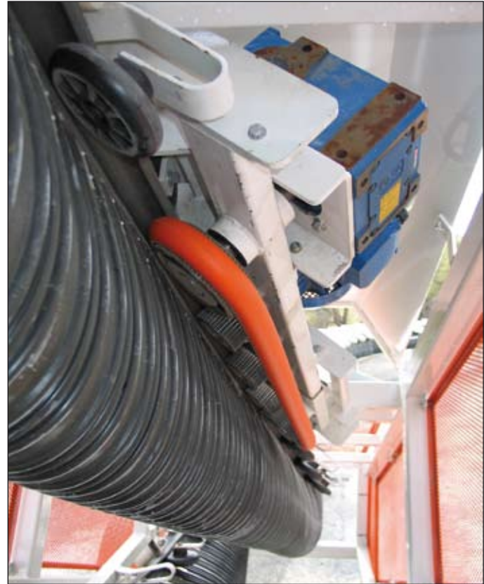
The conveyor uses multiple drives to distribute the loads along the length of the system. These drive units can be easily repaired or replaced when necessary.
